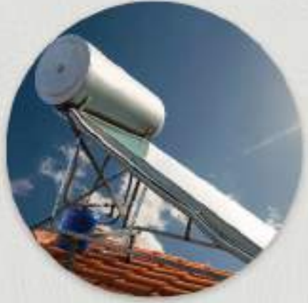
Solar Water Heater
